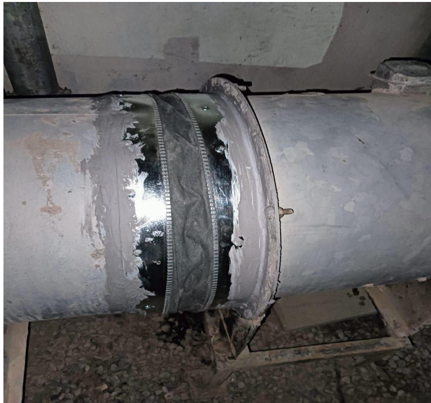
Kitchen Hood duct extensions
